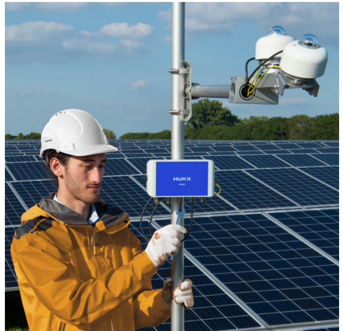
Figure 8 Two SR300-D1 pyranometers that are connected to the SPD01 Surge Protection Device. With the optional SPD01, you can upgrade surge immunity to level 4.
